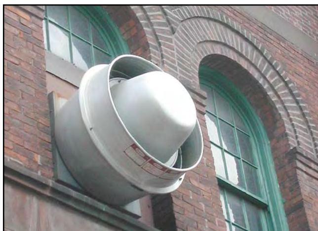
This installation does not meet clearance standards.
